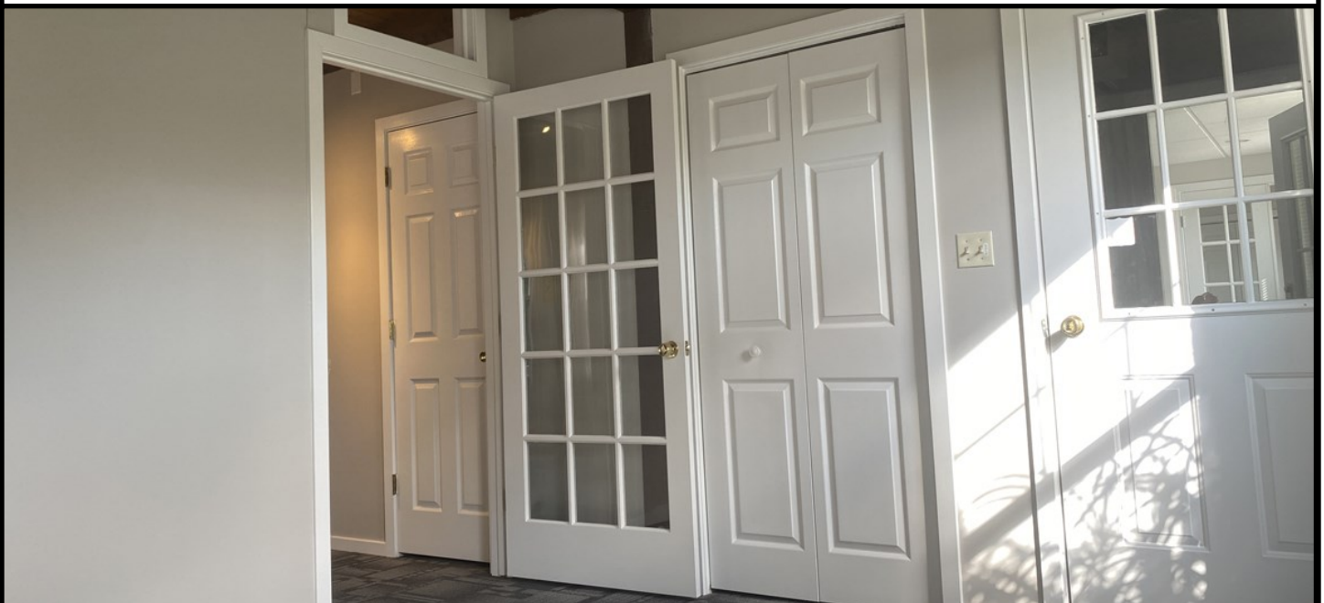
Above- Standing in the front office. To the right, straight ahead, is the door to the front foyer. Middle is the closet door. Left, the glass panel door, goes to the wide open room and the two bathrooms.
